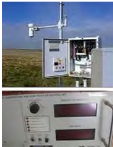
Figure 6-11: AN/FMQ-8 Temperature Dew Point Measurement Set, sensor and electronics on top and indicator on bottom.
