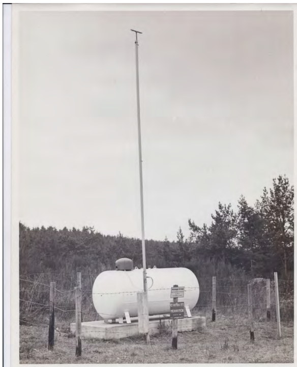
Figure 5-17: Manually activated CFDS at Hahn AB, Germany.
