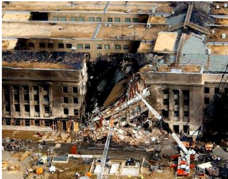
Figure 8-6: Pentagon damage from 11 Sep 2001 Terrorist Attack
